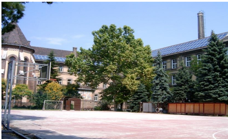
Fig.7. Photovoltaic system in Fasori Gimnázium in Budapest
